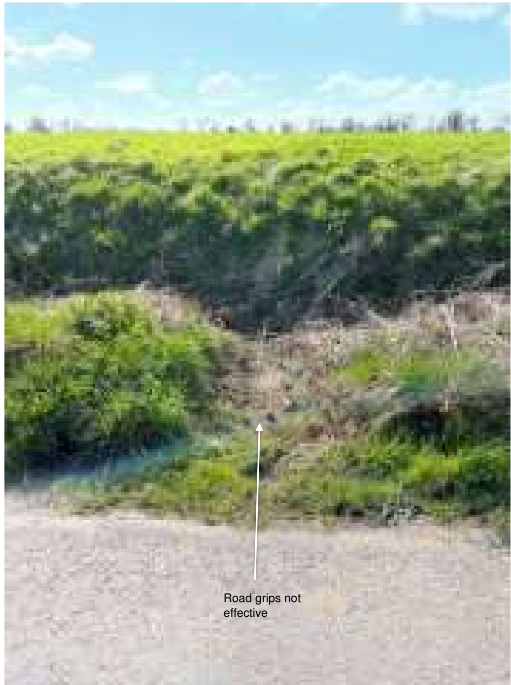
Along the length of Common Road the road grips should be checked to ensure they allow the fall of water from Common Road into the adjacent ditch. Several are not effective.
