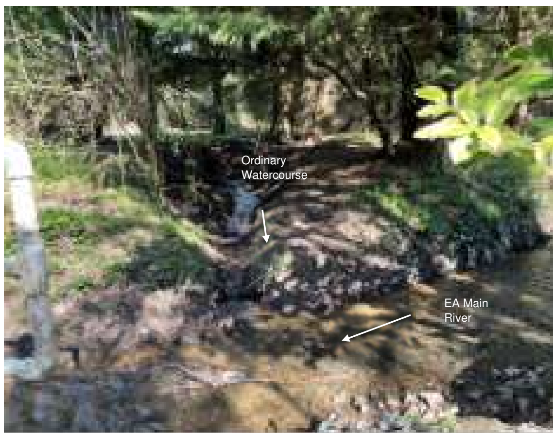
Point P5: Some minor maintenance and clearance required along the ordinary watercourse to the west of Church Road, within the grounds of Spa House, prior to reaching the Main River.
