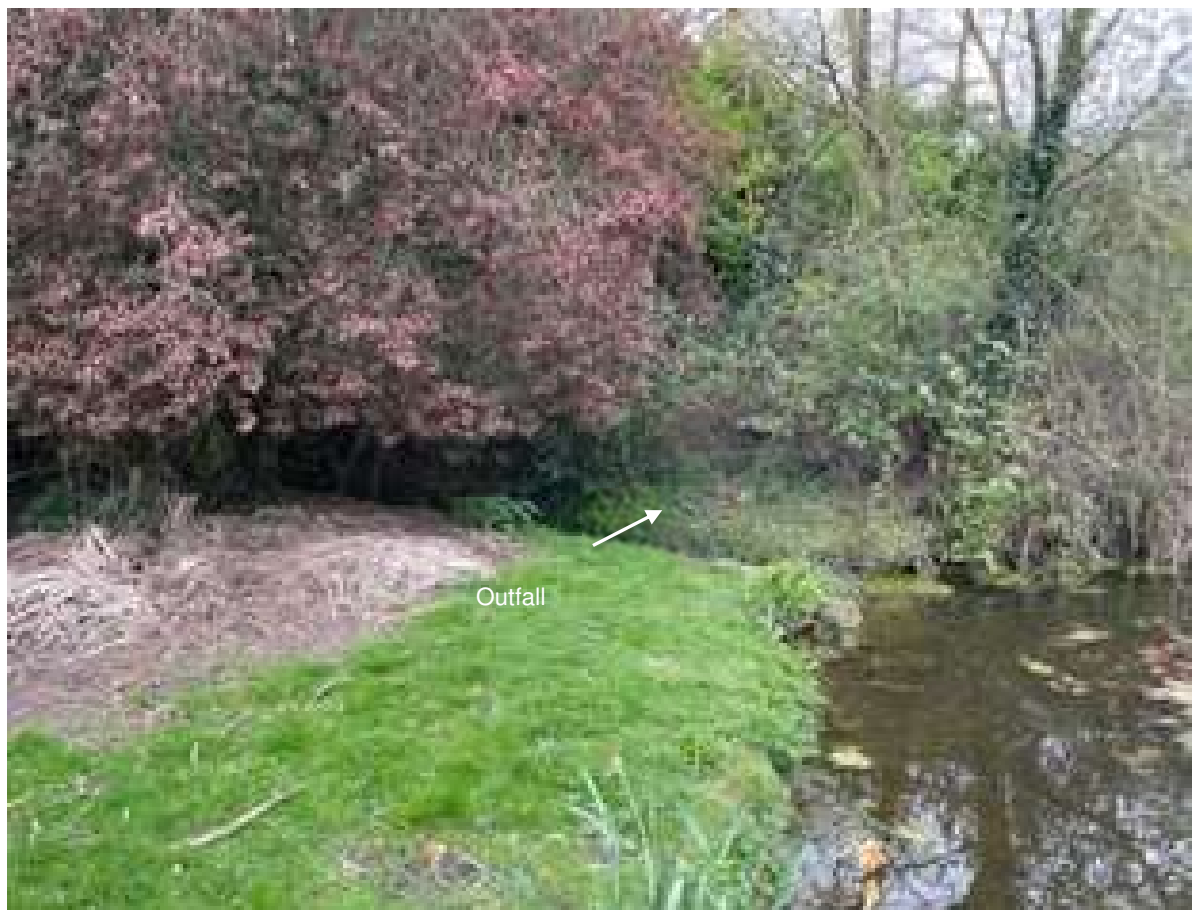
Point P12: Pond at Manor Farm with outfall into adjacent ditch along northern side of Common Road. The pond on the western side requires clearance.
