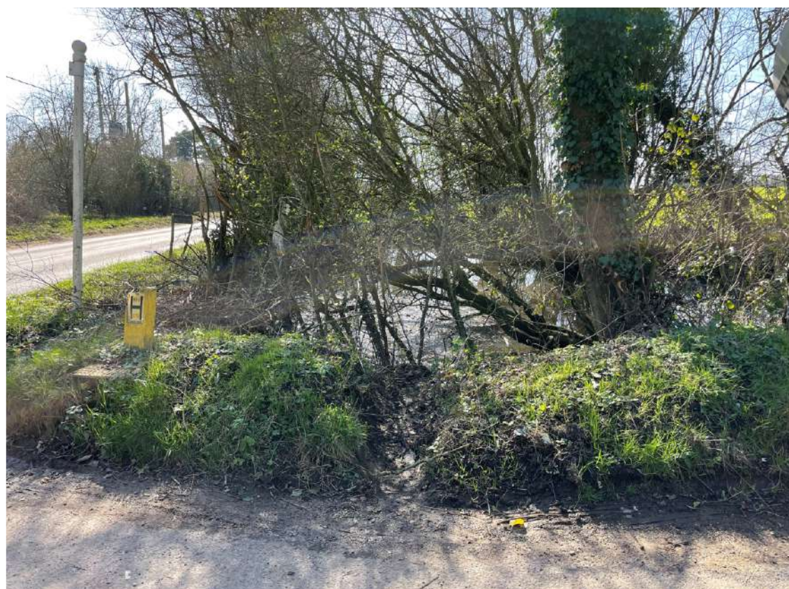
Point P3: Ponds to the north and south of Hall Road/east of Church Road require desilting and removal of fallen and overgrown vegetation to restore storage area for storm water prior to entering the culvert/ford under Church Road.
