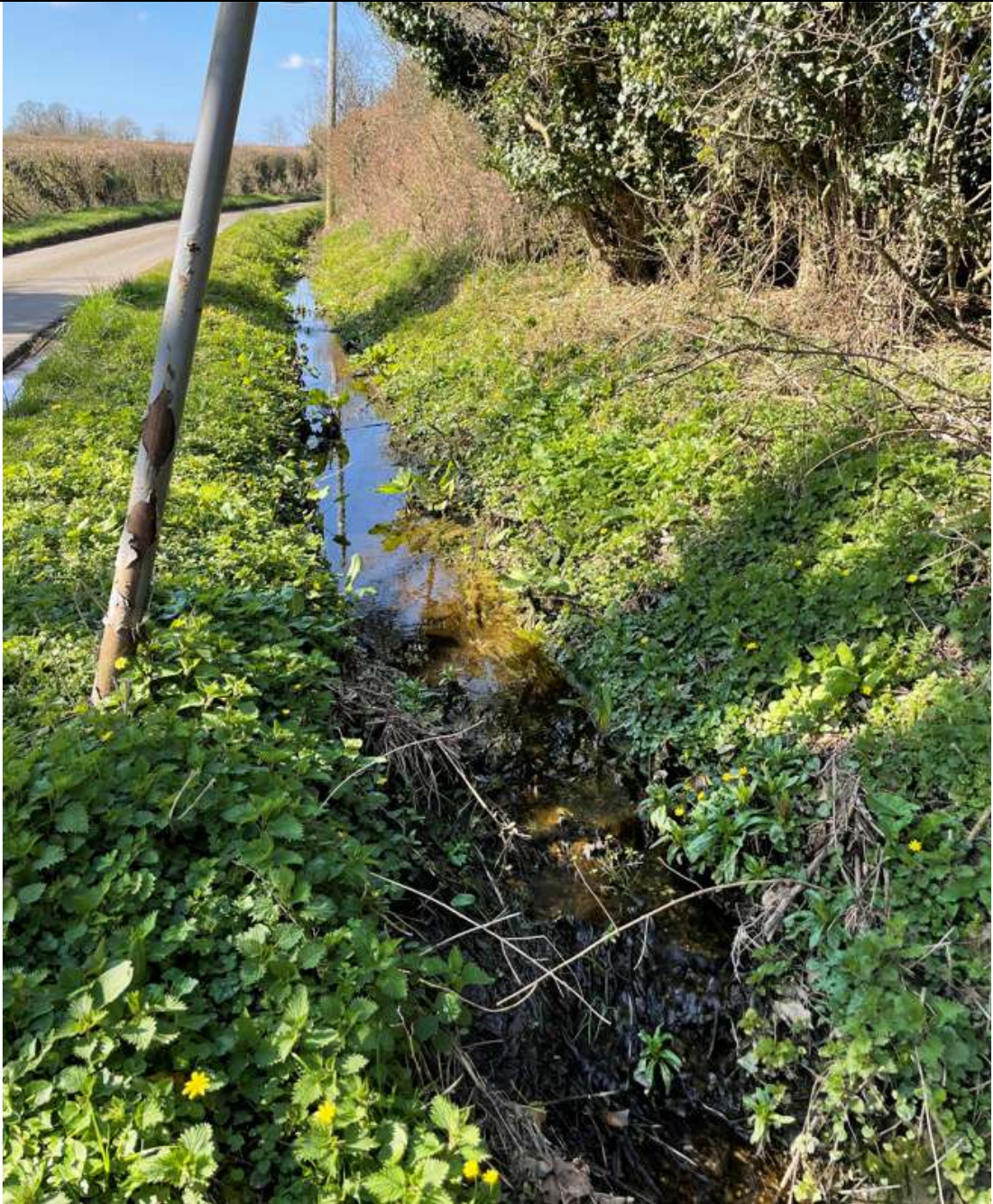
Point P1: Looking west along Hall Road from Church Road. Ditch network is silted up and requires clearance to improve flow towards the culvert under Church Road (ford in times of heavy rainfall).
